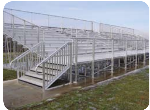
New bleachers installed at the Grandview Middle School football field, one of eighteen school improvement bond projects completed since July 2007.
