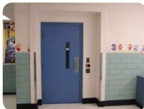
New wheel chair lift (from the cafeteria to the second floor) installed at Belvidere Elementary School in March, 2008.
